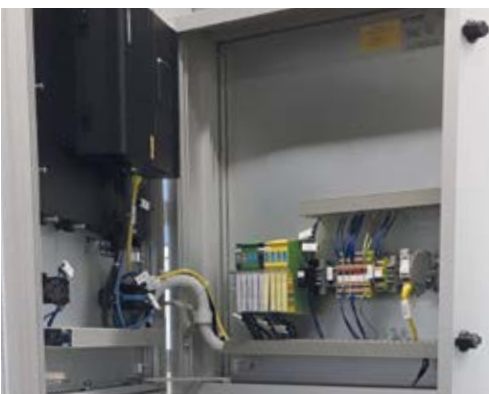
Assembly and wiring
